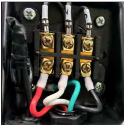
Figure 13. G8146Z motor junction box wiring.
