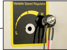
Figure 59. Variable speed dial wiring.
