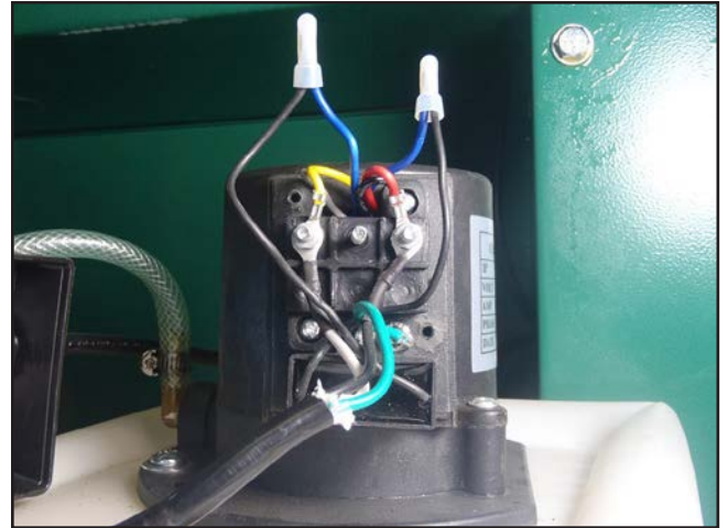
Figure 78. Pump motor (115V).
